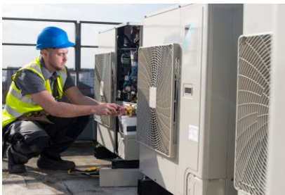
Heating, ventilation and air conditioning systems
